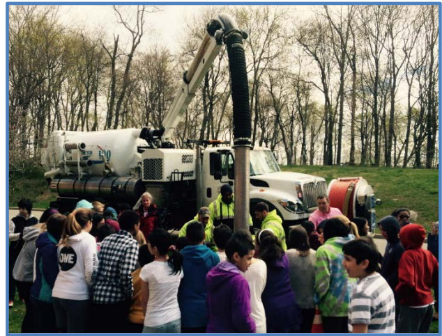
The Highways Department gives Stamford school children a demonstration of the City's procedure for cleaning the catch basins of its drainage system.
