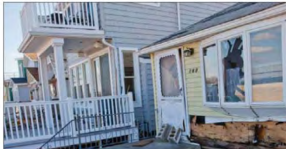
Thousands of dollars in flood damage can be prevented by building higher.
